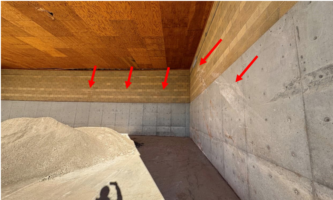
Figure 11. Salt discoloration on surface of north and east walls.
