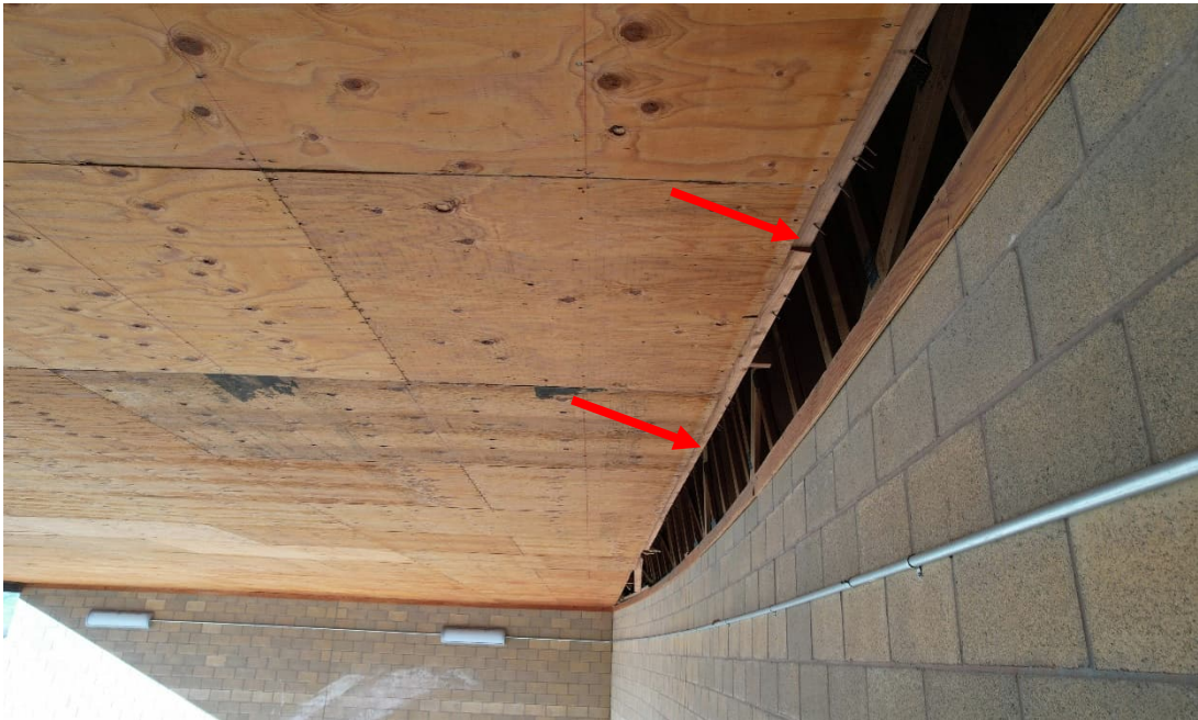
Figure 7. Outward displacement of north wall from ceiling finish.
