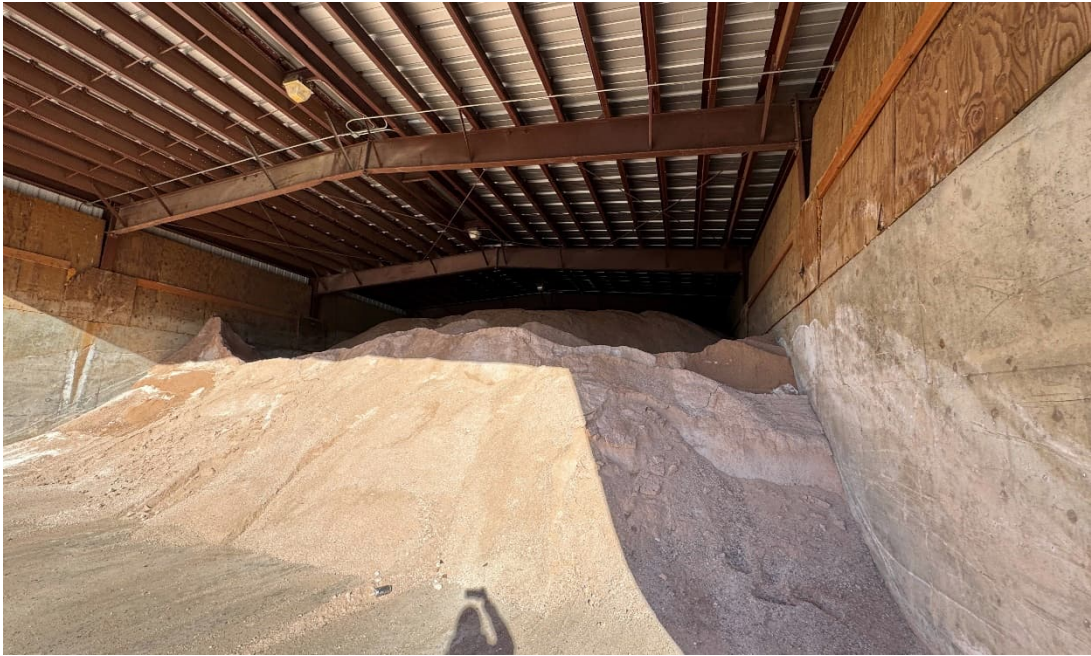
Figure 14. Interior of UDOT salt storage structure; salt bearing onto exterior walls.
