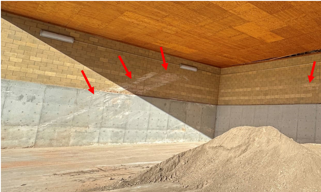
Figure 10. Salt discoloration on surface of west and north walls.
