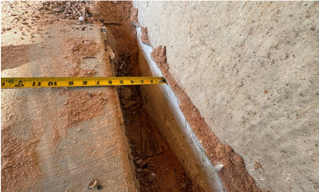
Figure 6. Outward displacement of north wall from floor slab.
