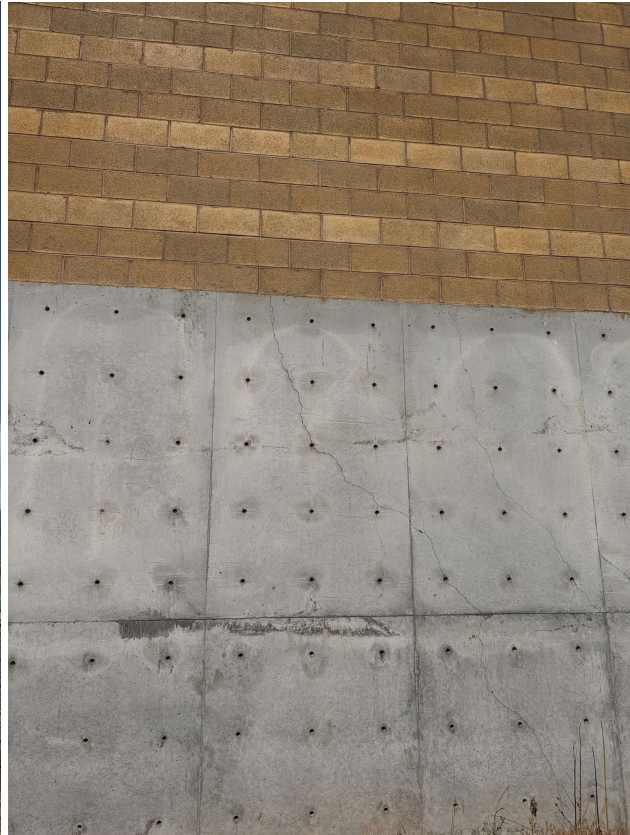
Figure 6: Cracking at middle of west side wall
